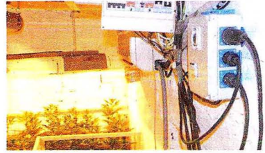
Automatic controllers available at hydroponics stores make it very easy to manage the grow room atmosphere.
