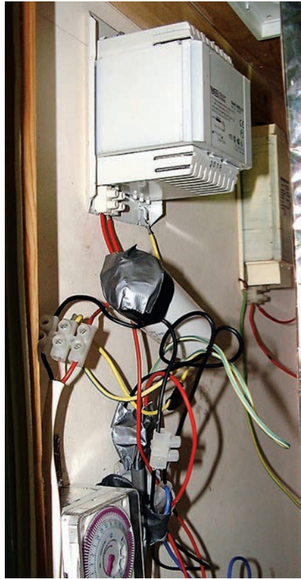
This ballast has been wired poorly. Good growers have well-organized electrical systems.
