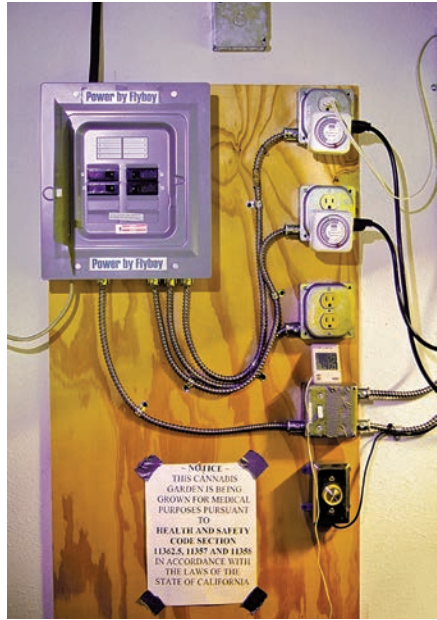
This complex wiring system required a professional electrician to complete.
