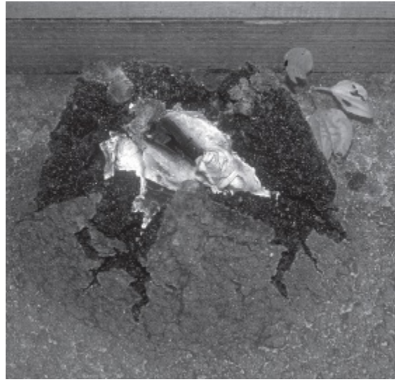
Mushrooms breaking through asphalt
