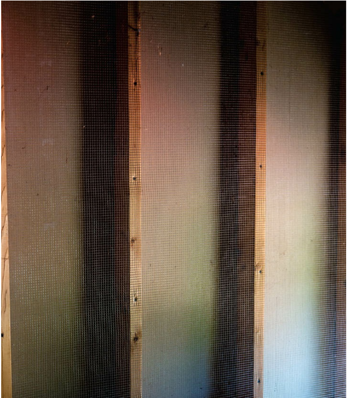
Rodent-proof wire-mesh screening surrounds the outside walls, floor, and ceiling of Avena's drying rooms.
